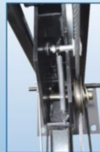
Cable safety system
